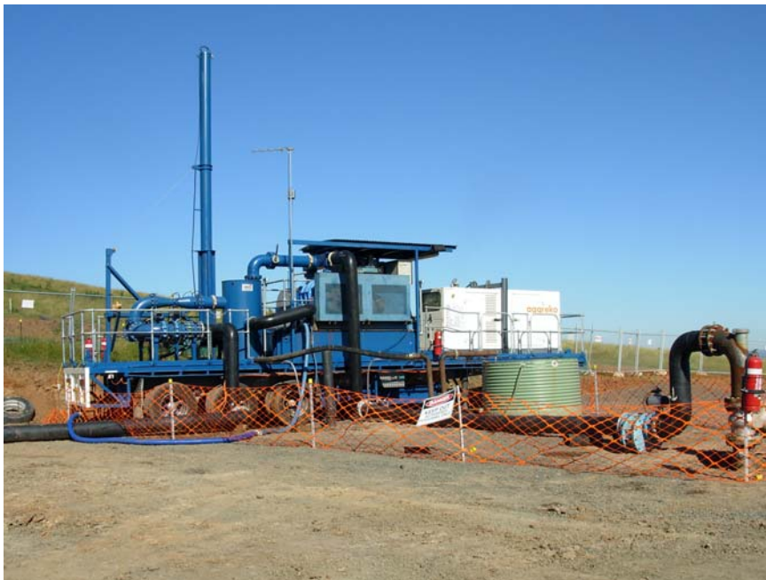
Photo 2. Liquid Ring Vacuum Pump at Appin, NSW
