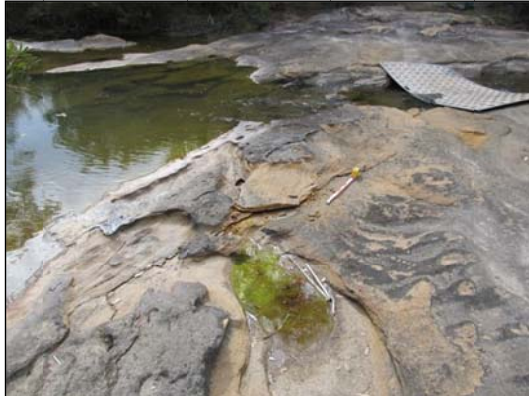
Plate 1: minor cracking observed within the base of the Georges River at Rock Bar 41
