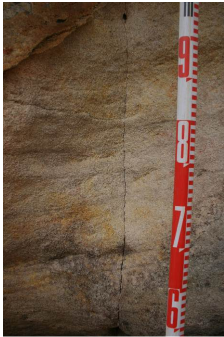
Baseline record - Vertical joint plane prior to longwall mining, located below the main art panel
