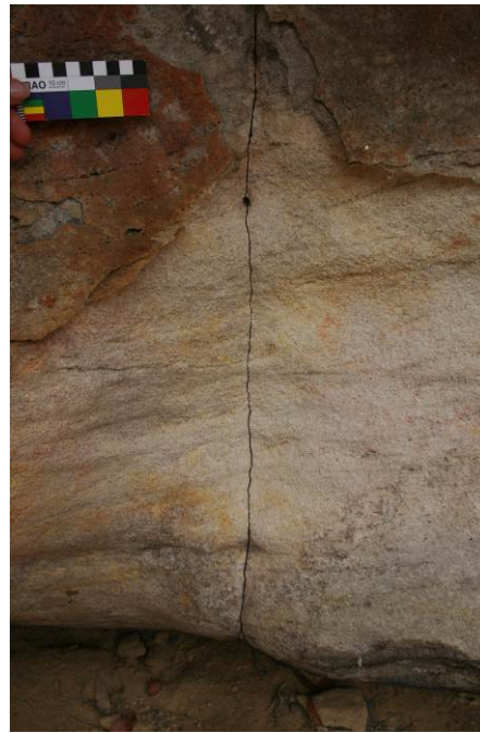
Post Longwall 6 record (2 February) - Vertical joint plane has begun to separate
