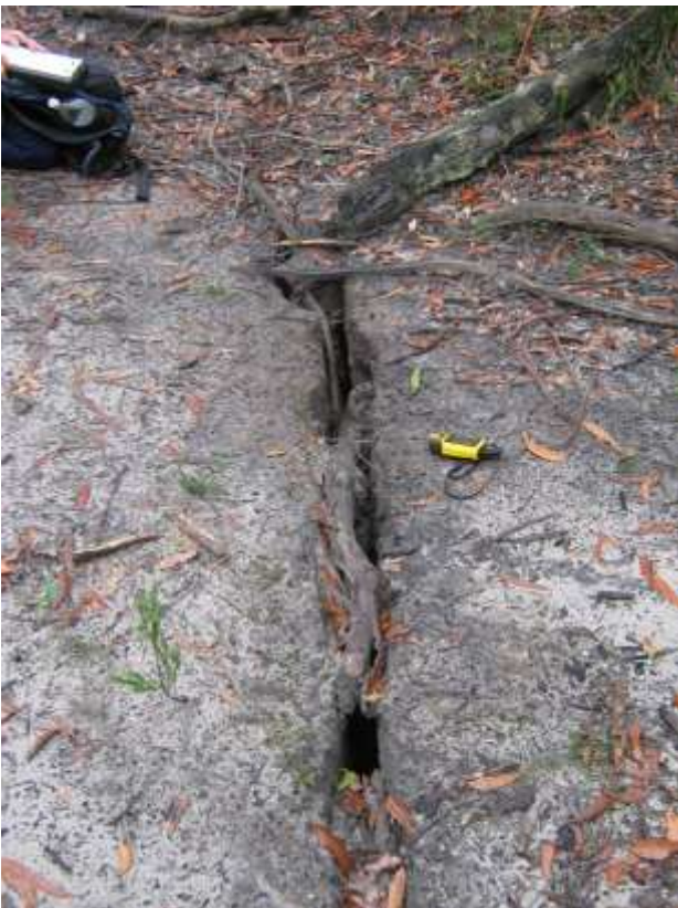
Plate 3: Soil cracking and observed exposed tree roots..
