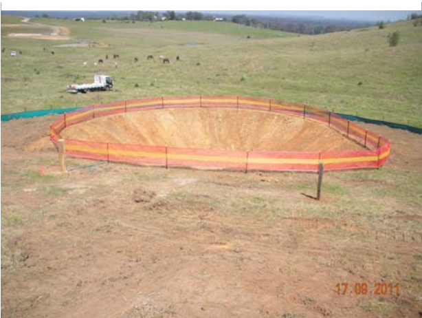
Figure 4. Construction site runoff is captured in sedimentation ponds where it can be managed.
