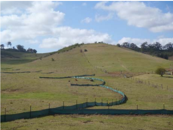
Figure 3. Sediment fences have been installed to filter any runoff from construction activities.
