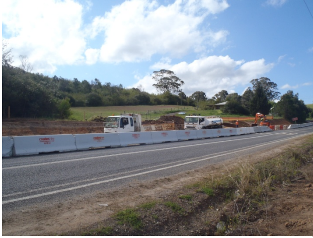
Figure 2. Stage 4 traffic management controls included the installation of barriers on the far (eastern) side of the road. Lane markings were adjusted to address the new alignment.
