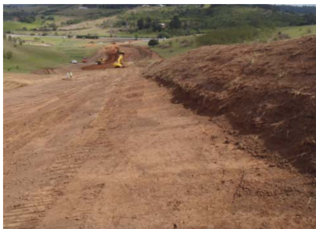
Figure 8. Topsoil has been separated and stored above the proposed banks. Once the banks are completed the topsoil will be utilised to enable the banks and road verge to be re-grassed.
