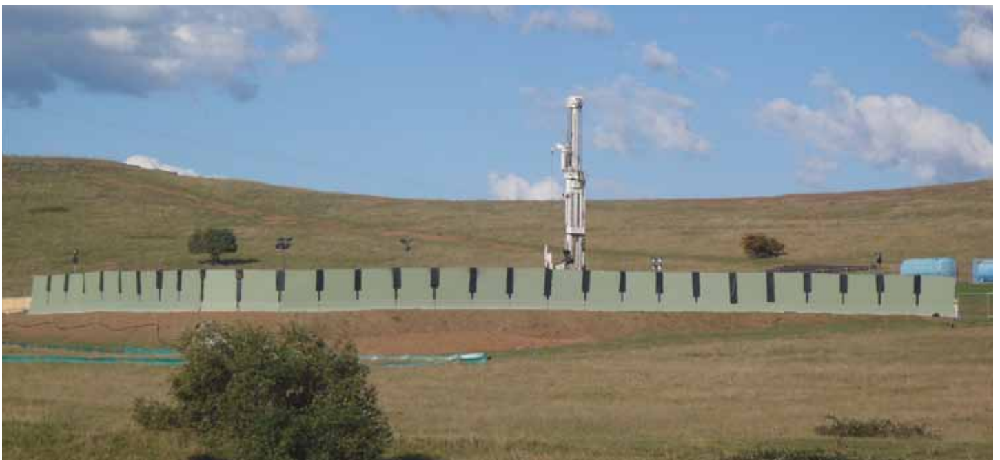
Illawarra Coal has been conducting surface goaf gas drainage works on Company-owned property in Douglas Park in order to create a safe working environment underground.
