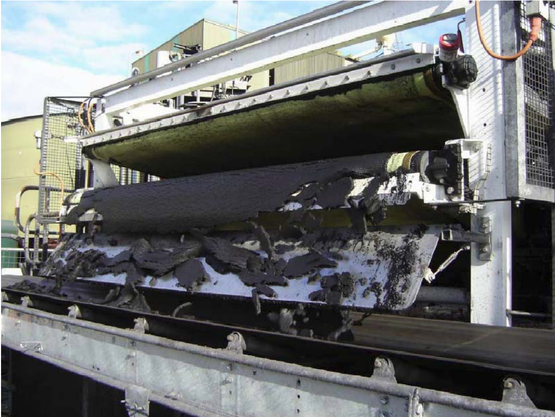
Figure F-5 Belt press filter in operation in a Hunter Valley coal mine operation
